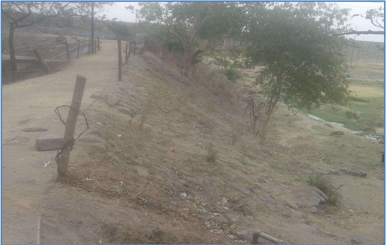
Picture 3 - Stone Pitching/embankment at Kari Jore
