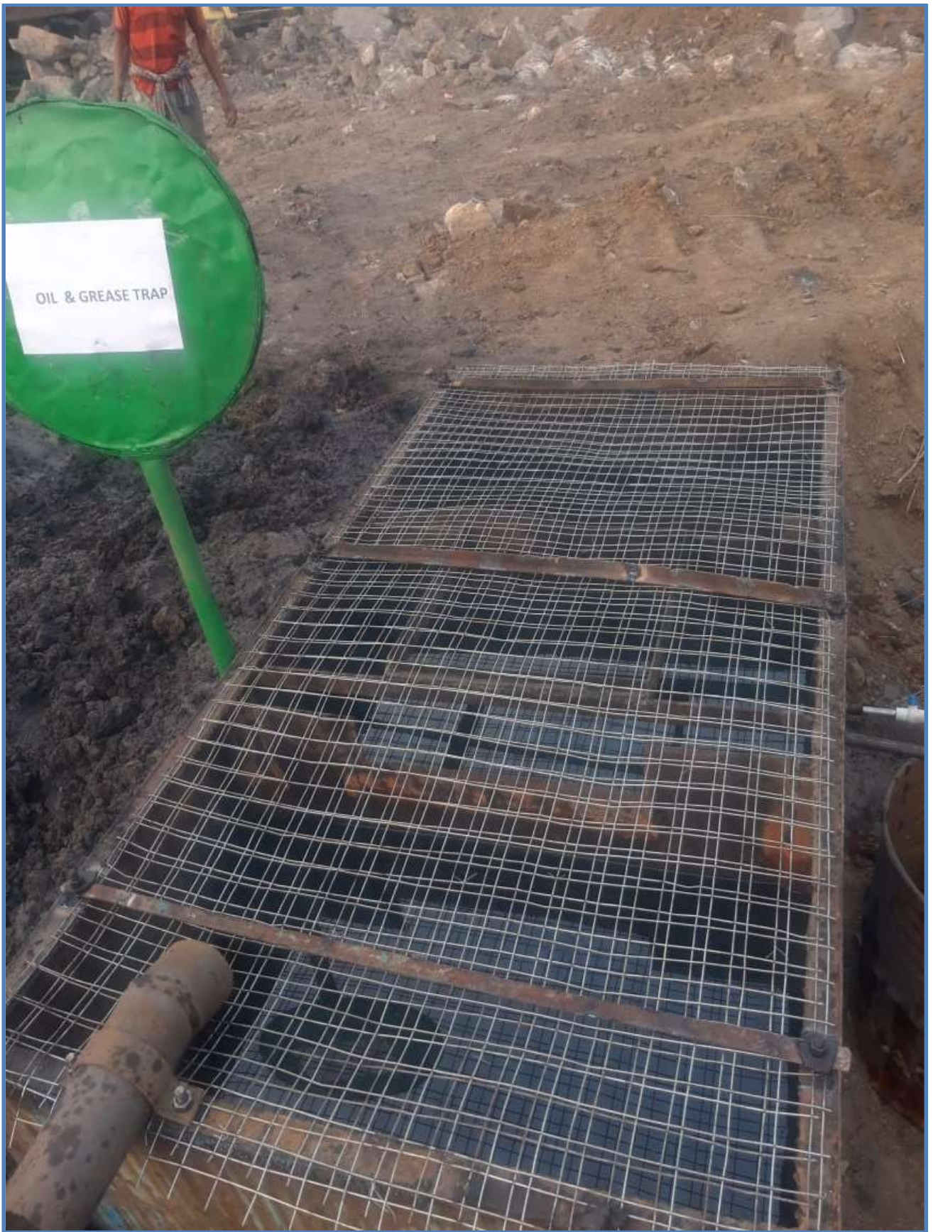
Picture 5 – Oil & Grease Trap
